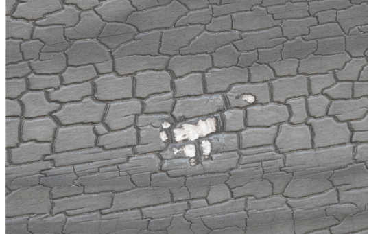
Close-up of damaged SSB Gator®
