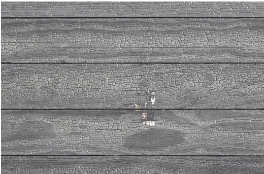
Damage from a ladder - scraped SSB Gator®
